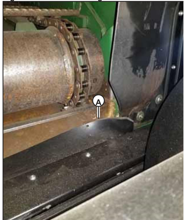
Figure 4.14: Too Large Transition Frame Seal
