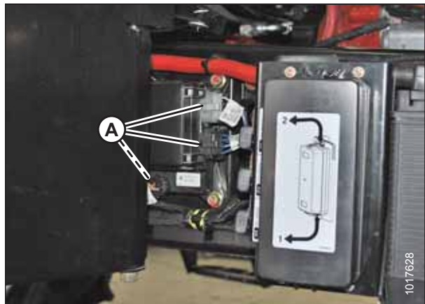
Figure 1.19: Chassis Relay Module
