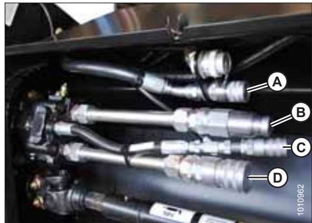
Figure 3.79: A40D Hose Connections – 5.4 m (18 ft.) Header Shown
