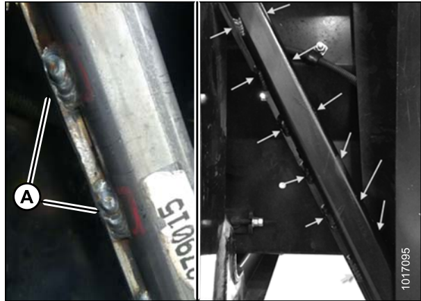
Figure 3.13: Weld Locations along Edges of RH Cross Brace Tube
