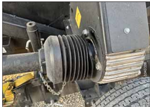
Figure 3.3: Main Driveline Guard – Incorrectly Seated
