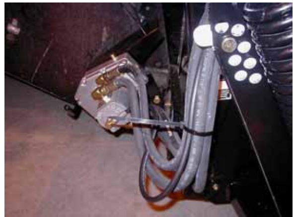
PUMP IN WORKING POSITION (FIXED SPEED FEEDER HOUSE)
