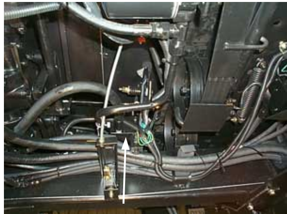
HEADER CONTROL VALVE
